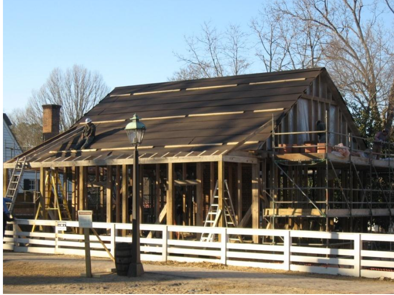
In the process of reconstructing the Richard Charlton's Coffee House in 2009 at Colonial Williamsburg-Photo taken by Alyssa Holland
